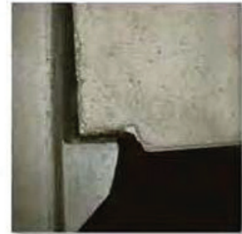
This concrete girder rests on the ledge that is assumed to act as a smooth contacting surface.
