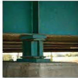
The rocker support for this bridge girder allows horizontal movement so the bridge is free to expand and contract due to a change in temperature.
