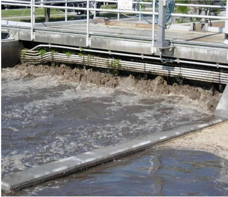
Mechanical aeration at Waste water treatment plant
